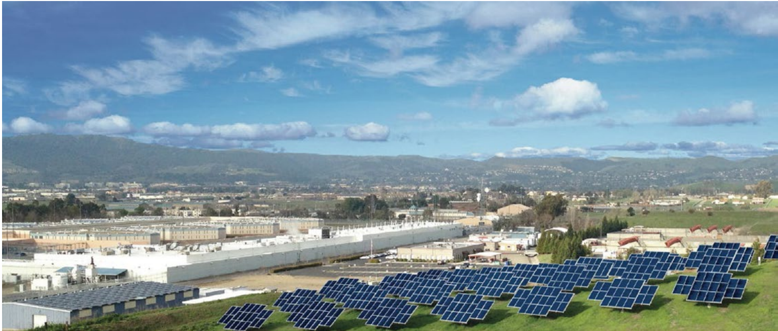
Solar panels help provide the Santa Rita Jail with renewable energy via the jail's microgrid.
