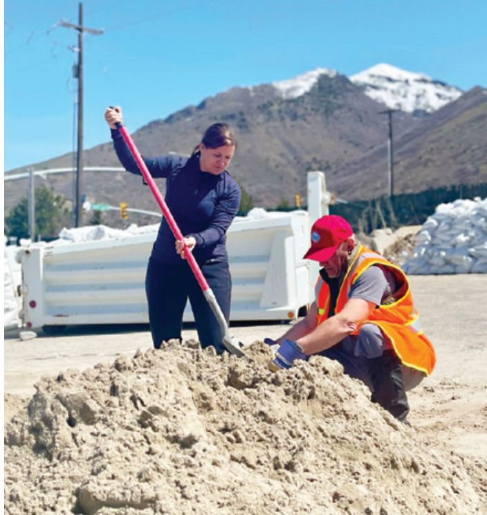
Salt Lake County, Utah Mayor Jenny Wilson shovels sand into sandbags to prepare for flooding. Photo courtesy of Salt Lake County
