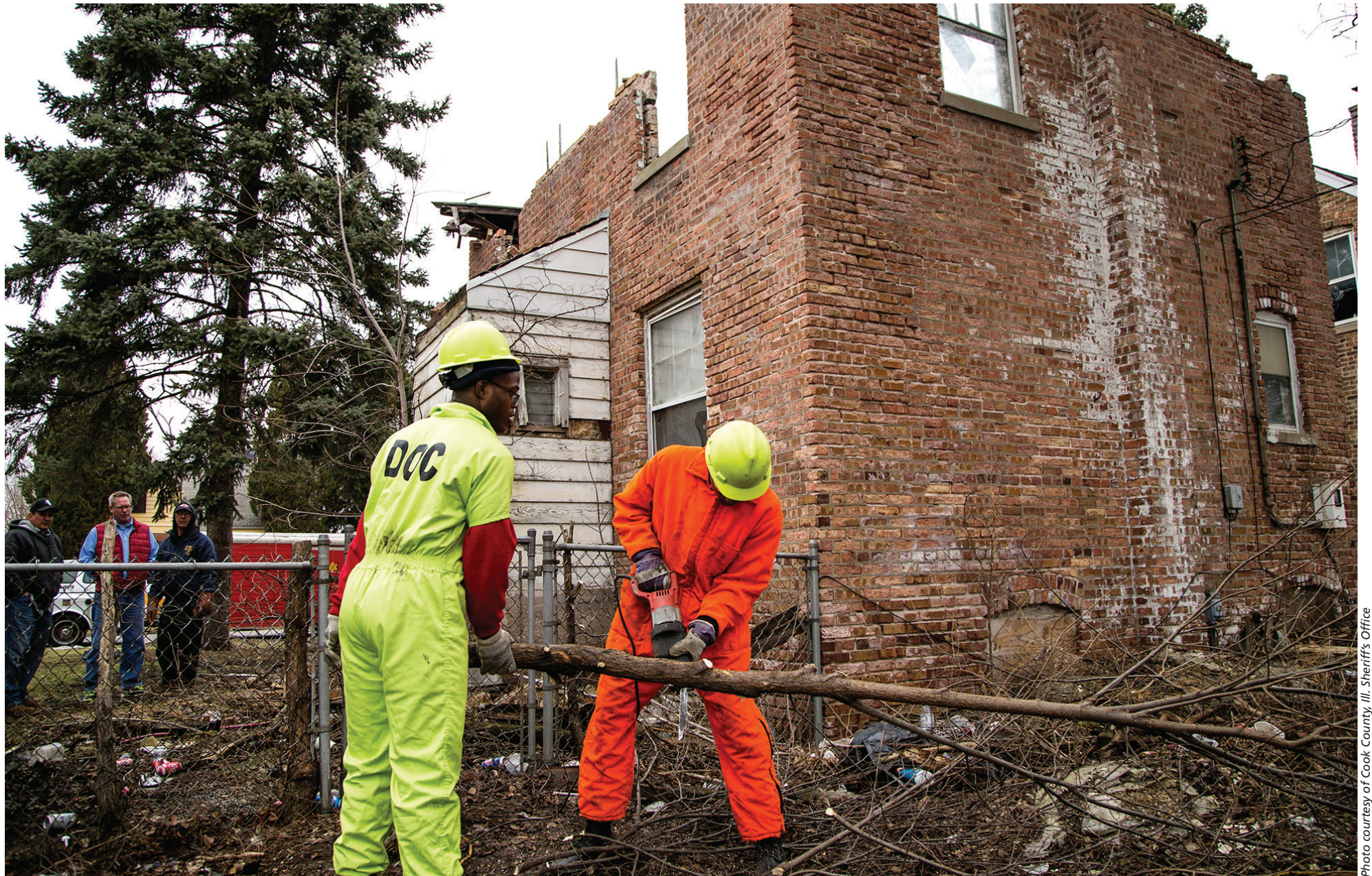
Inmates and house-arrestees do site maintenance along with building deconstruction in the Cook County sheriff's RENEW program.
