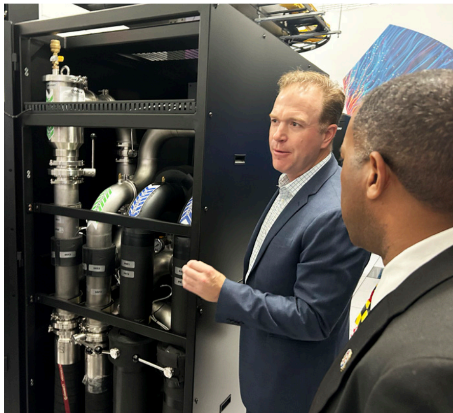
An associate with Digital Realty shows county officials the cooling system in one of its Loudoun County, Va. data centers in October 2024. Photo by Charlie Ban
