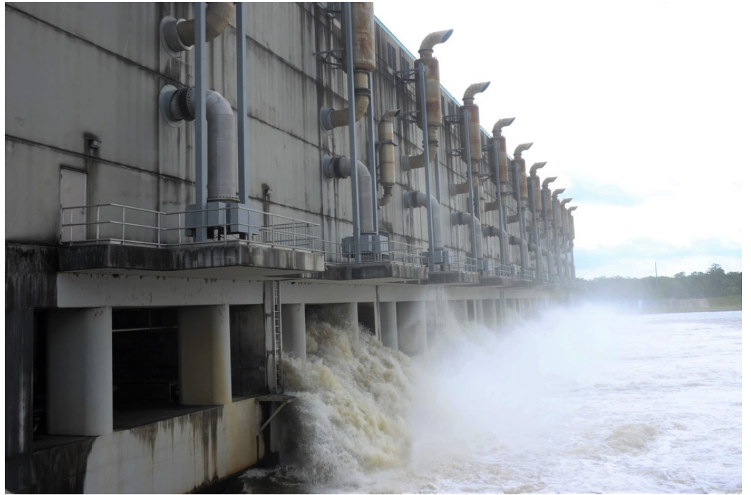
West Closure Complex in Belle Chasse, La., during a pump test. It serves as the world's largest drainage pump station, designed to protect against storm surges. Photo by Ryan Labadens, U.S. Army Corps of Engineers
