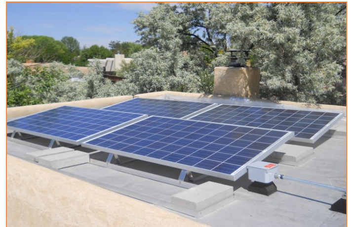
Ballasted (weighted) PV system.
