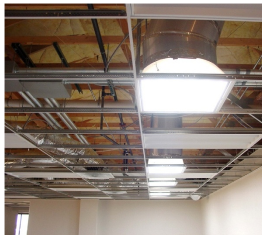
Solar tube lights installed in Mohave County buildings.
