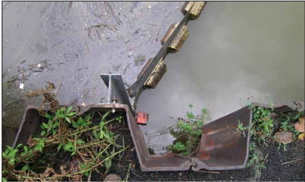
Debris and oil often seen along the Cuyahoga could be reduced by LID technologies.
